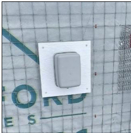
Single Radio Installation on a New Home
