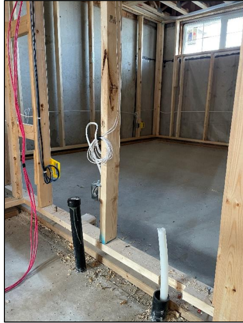
Cable Coiled at Meter Location
