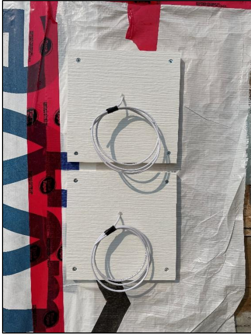
Cable coiled at Radio Location (2 Radios)
